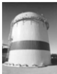
Digester at BTA facility in Newmarket, Ontario
