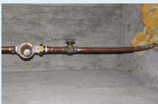
Make sure your family knows where the emergency water shut off is located inside your home!
