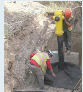
Construction crews assemble and install a fire hydrant as part of the new water system to service Upper Fintry, Shalal Road and Valley of the Sun.
